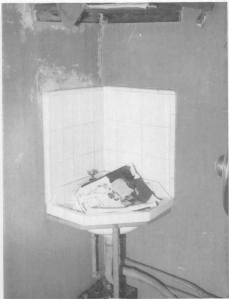
A corner of an autoclave room. The room was in a state of disrepair and the wash-hand basin used as a receptacle for refuse
